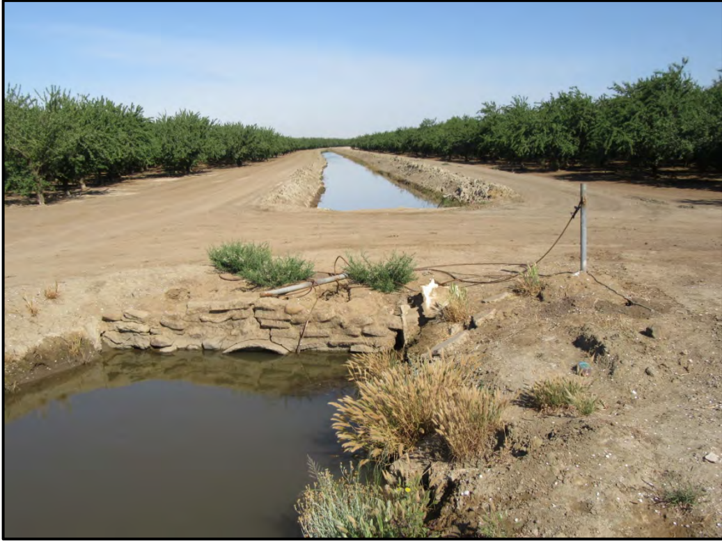
West Stanislaus Irrigation District Lateral that will be crossed by the pipeline, looking northwest; 05/30/17. The pipeline may be trenched under the culvert to minimize disturbance to the lateral.
