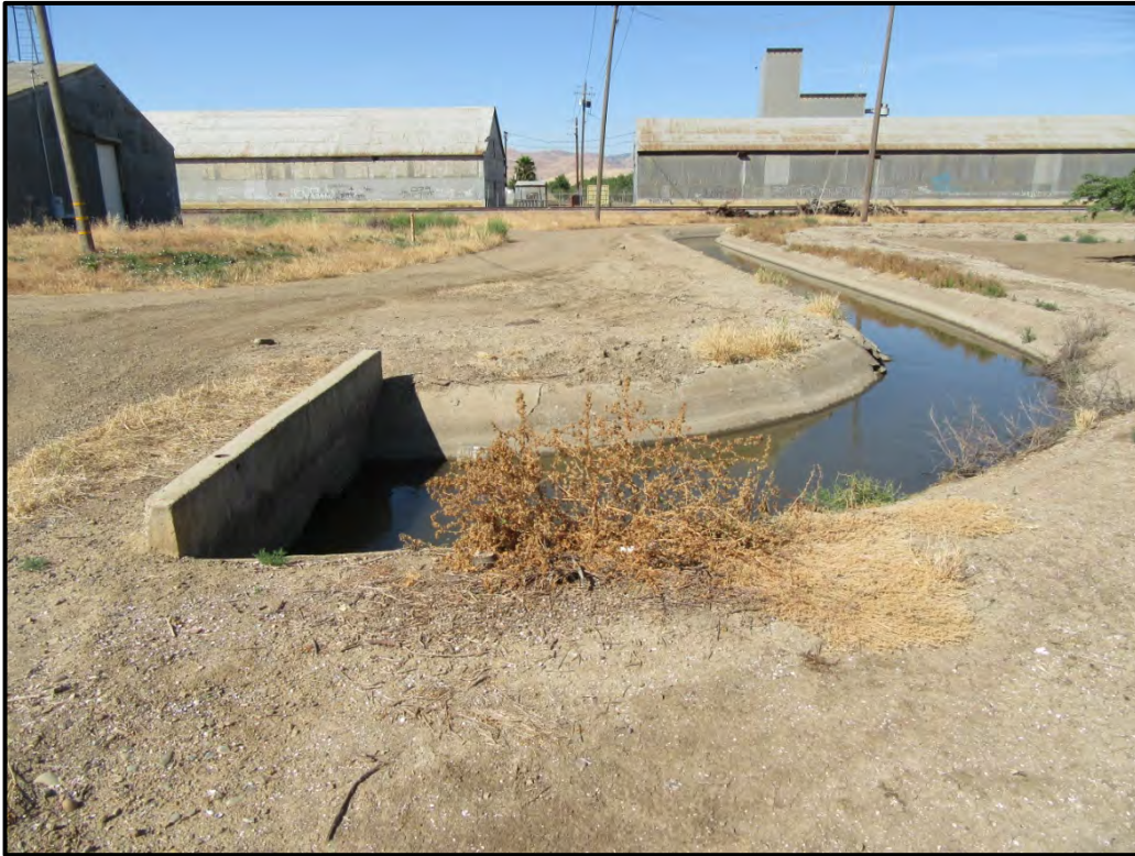
Concrete-lined irrigation lateral just east of the railroad tracks in Westley; 05/30/17. The pipeline will be bore & jacked under this lateral and under the railroad tracks.
