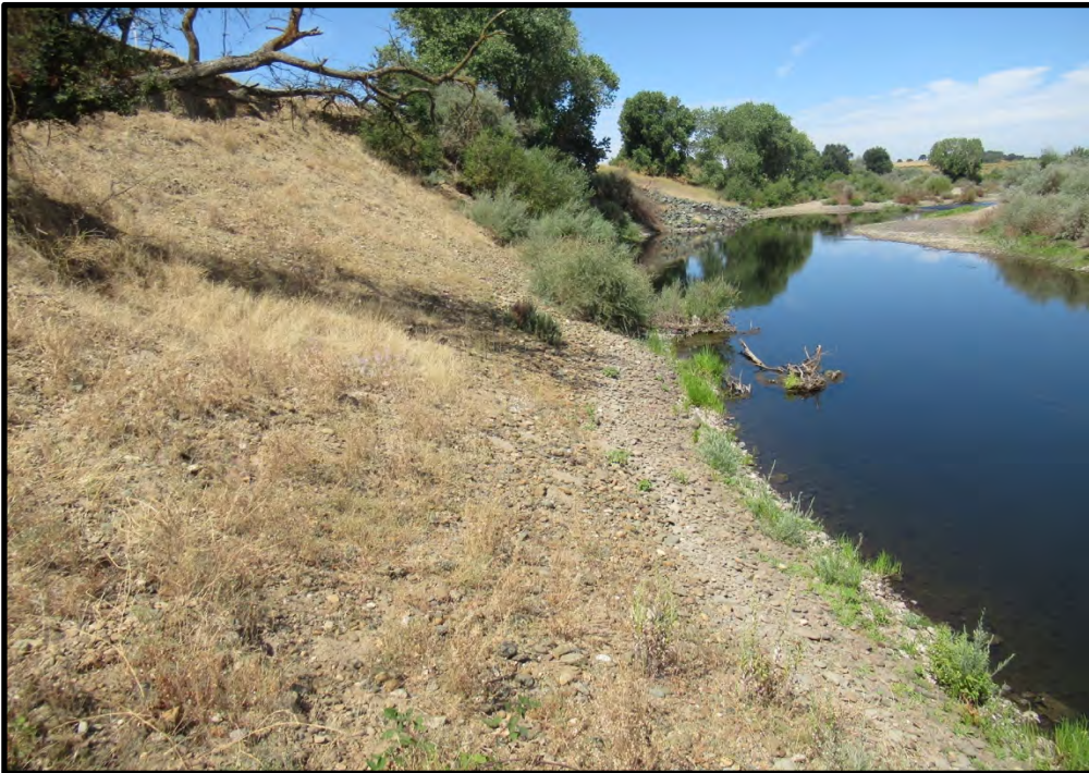
Meiss Road Upstream, looking west from the east end of the repair site; 08/05/19.
