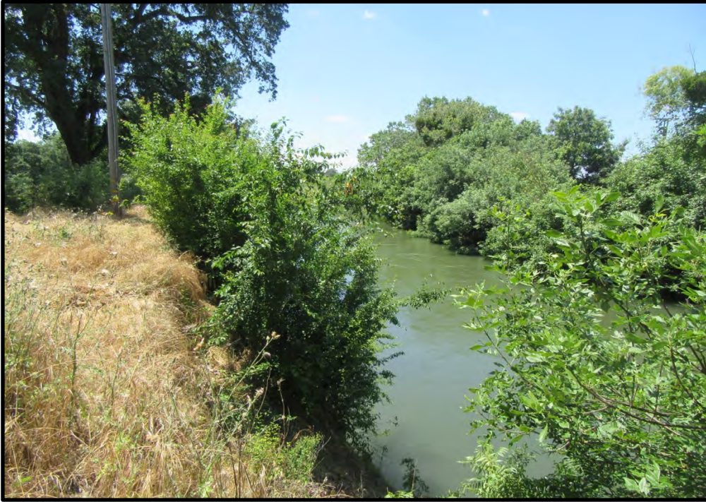
Eroding bank at the Cosumnes Road Downstream site, looking southwest from the north end of the work area; 05/27/19.
