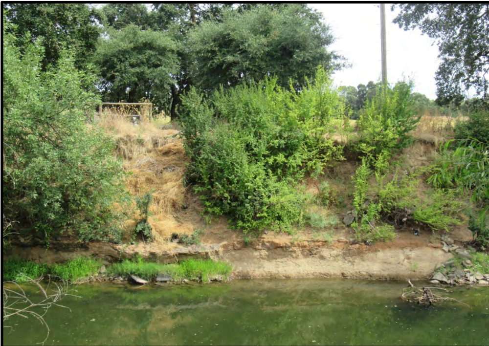
View of the eroding bank at the Cosumnes Road Downstream site, looking southeast from across the Cosumnes River; 08/05/19.
