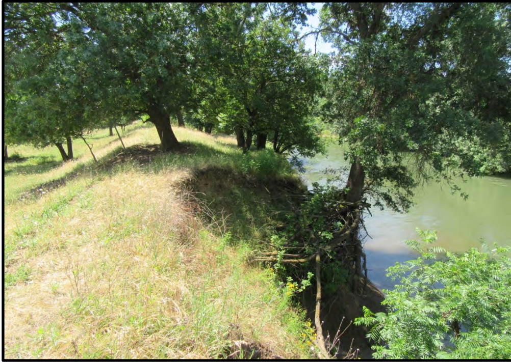
Tree hanging on to the bank by its roots in the south part of the Freeman Road site, looking south; 05/27/19.
