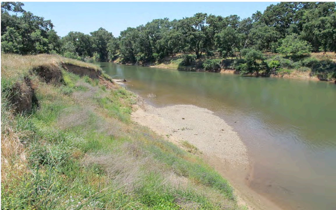
Figure 2-A. South bank at the Fig Road - Downstream repair site, view looking downstream. Again, severe signs of erosion near the top of levee and a shallow gravel bar that extends to near mid-channel.
