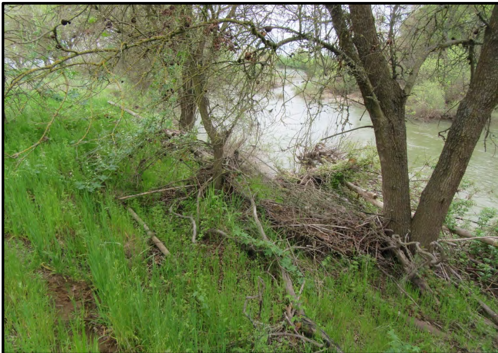
Mile Marker 19, looking northeast; 04/04/19. Several trees and shrubs need to be removed at this site to accomplish the repairs.
