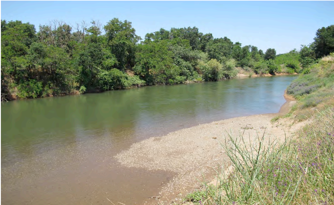
Figure 1-A. South bank at the Fig Road - Downstream repair site, view looking upstream. The bank shows severe signs of erosion with sheering at the top of the levee. Near shore gravel bar appears to originate from levee spilling into channel via erosion processes.
