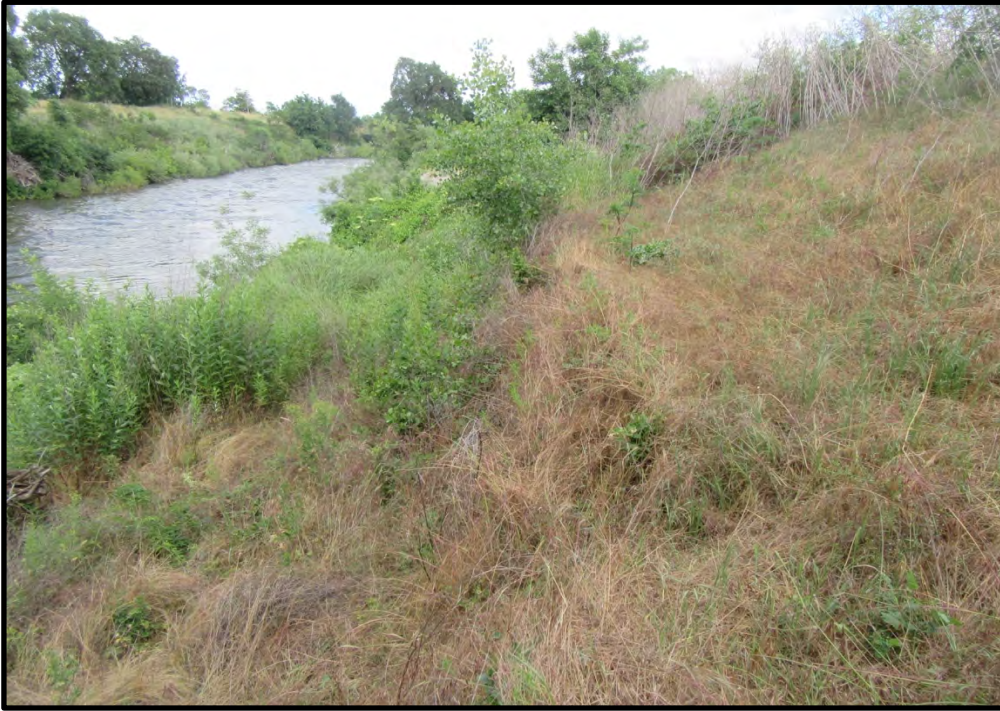
Meiss Road Downstream, looking northeast at the eroded slope; 05/17/19.
