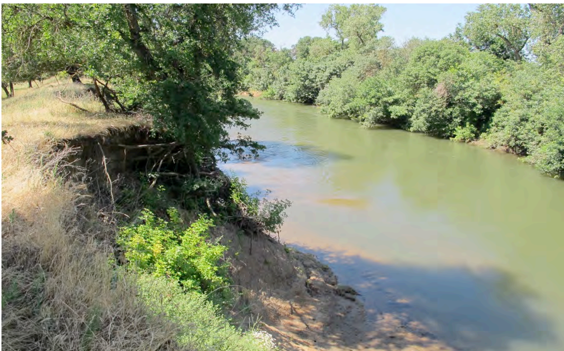
Figure 5-A. South bank at the Freeman Road repair site, looking downstream at of the top of the levee showing similar effects of erosion as other sites, resulting in steep, unprotected banks with clay substrate shelf and little shaded riparian area.
