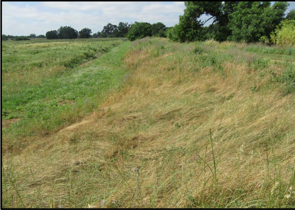
Fig Road Upstream, looking southwest at the landside levee slope; 05/24/19. Work at this site is limited to adding soil to the landside of the levee.
