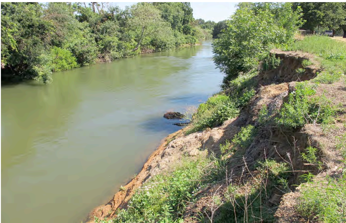
Figure 3-A. South bank at the Cosumnes Road – Downstream repair site, view looking upstream. Again, severe signs of erosion near the top of levee. A clay substrate shelf has begun to form at the nearshore with very little emergent vegetation or shaded riparian area.
