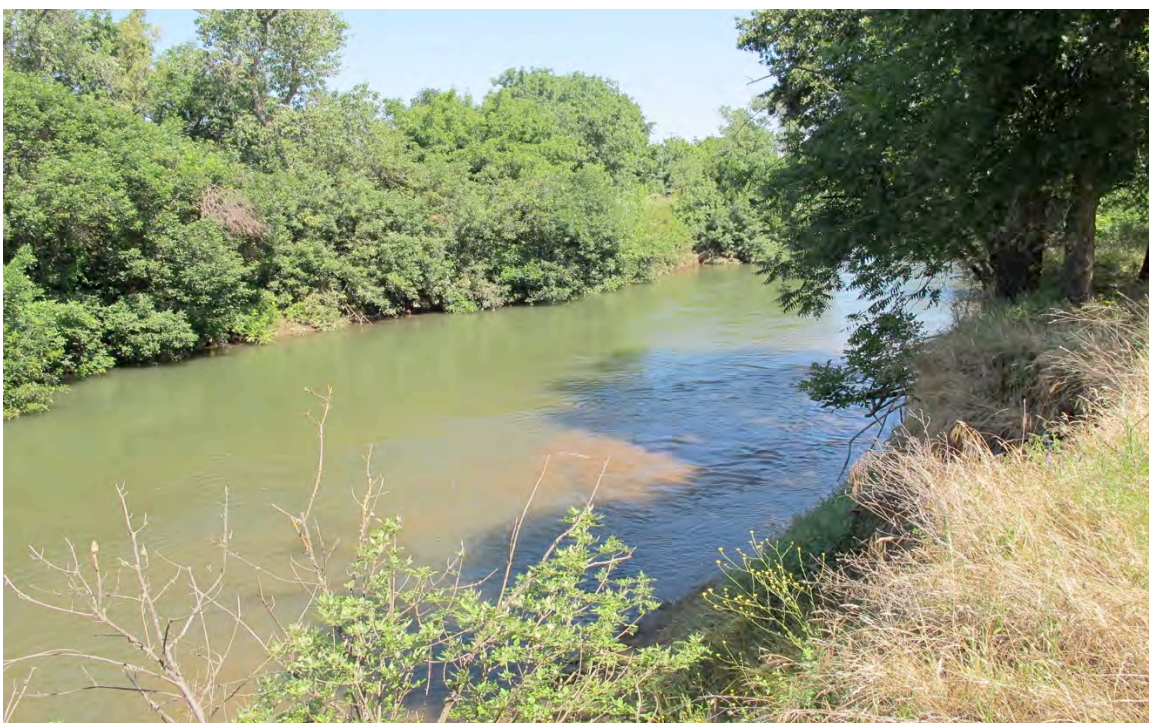
Figure 6-A. South bank at the Freeman Road repair site, looking upstream at of the levee illustrating the extent of the clay substrate shelf and similar erosion issues.
