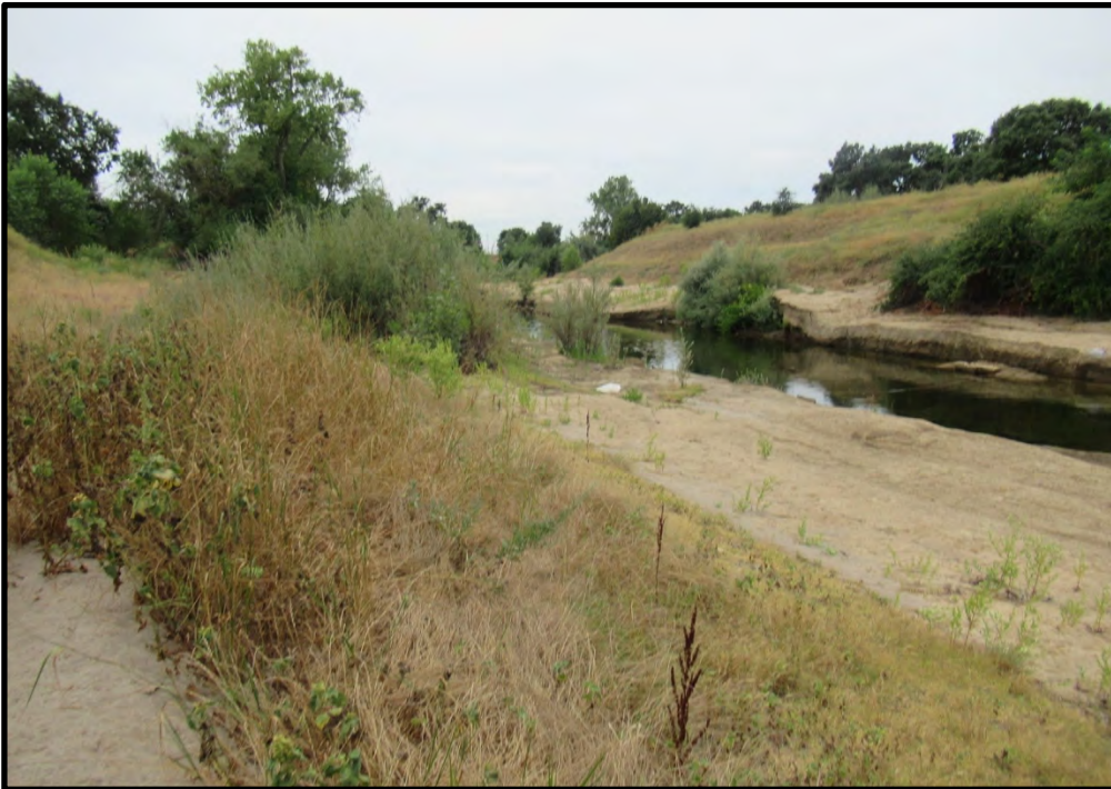
Keating Road site, looking south from the central part of the repair site; 08/05/19.
