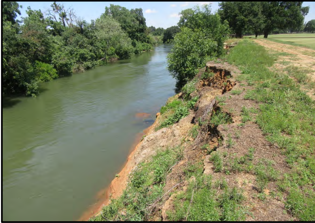
Cosumnes Road Upstream, looking northeast at the eroded levee slope; 05/27/19.
