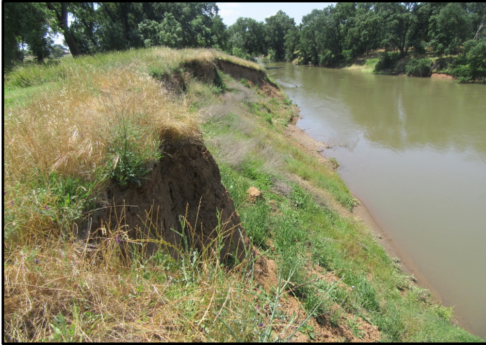
Eroding bank at the Fig Road Downstream site, looking southwest from the north end of the work area; 05/24/19.
