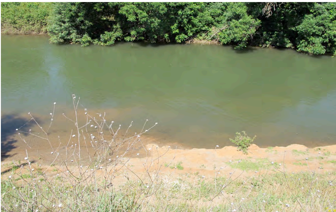
Figure 4-A. South bank at the Cosumnes Road – Downstream repair site, view downhill of the top of the levee showing the extent of the clay substrate shelf intrusion into the main channel.
