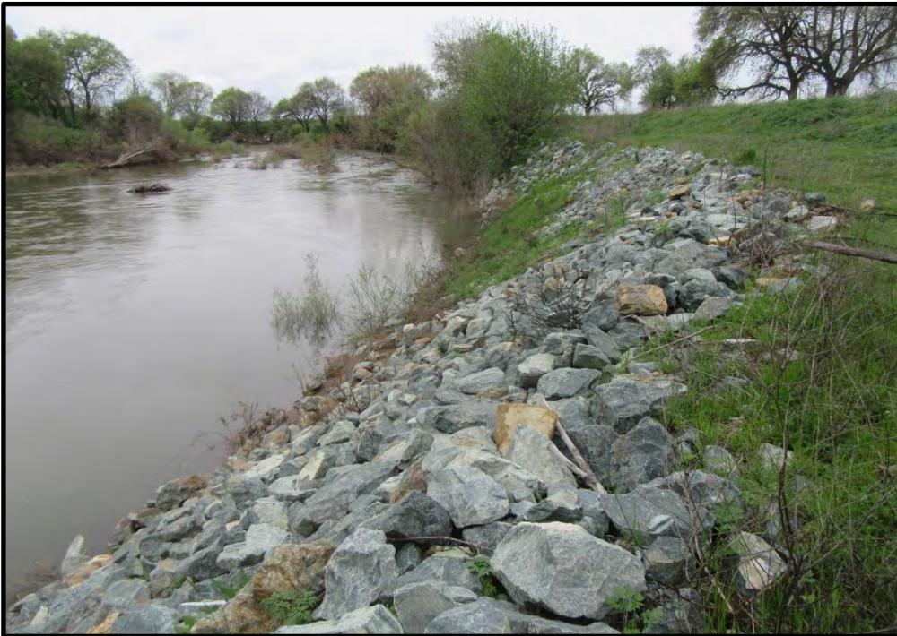
Rocked levee slope a few hundred feet upstream of the Mile Marker 19 site, looking northwest; 04/04/19.
