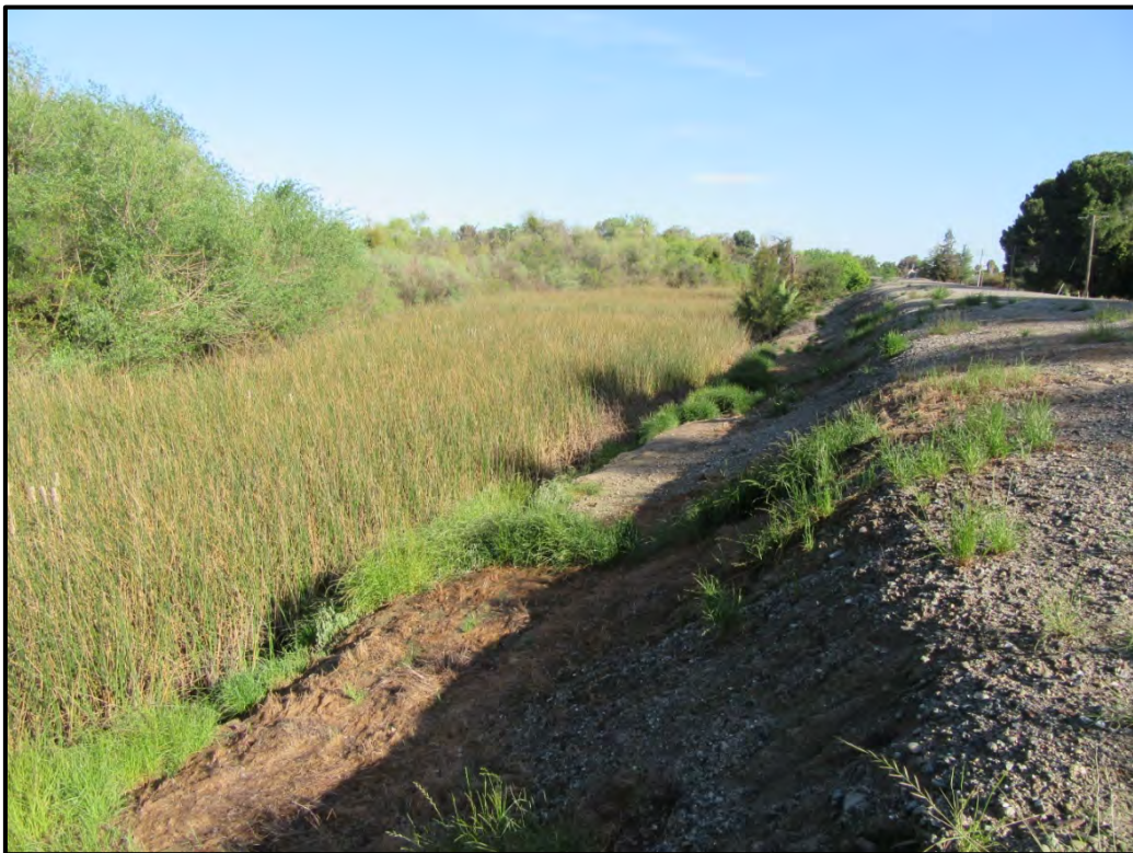
Waterside levee slope in the central part of the project site, looking northwest from Station 43+50; 04/21/17.
