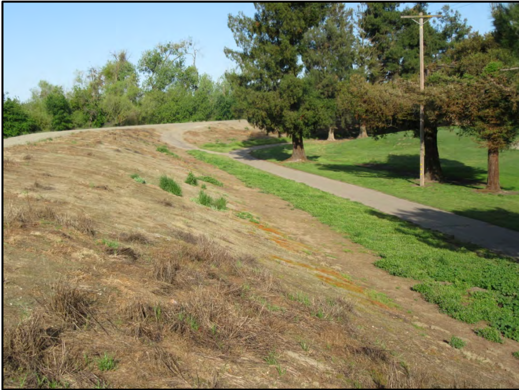
Landside levee slope at the east end of the project site, looking west from Station 38+00; 04/21/17. The Van Buskirk Golf Course is located just north of the levee.
