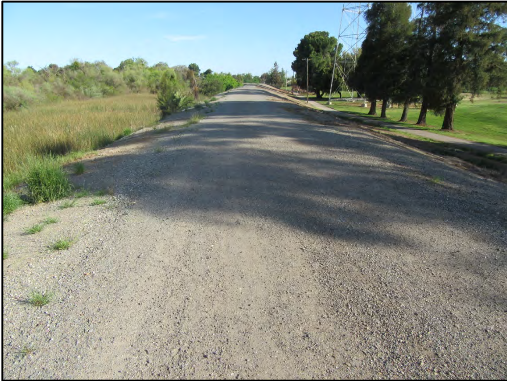
Levee crown and slopes in the central part of the project site, looking northwest from Station 43+50; 04/21/17.
