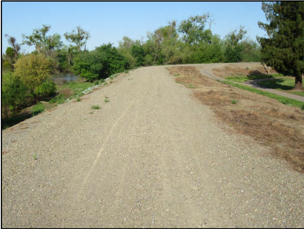
Levee crown and slopes at the east end of the project site, looking west from Station 38+00; 04/21/17.
